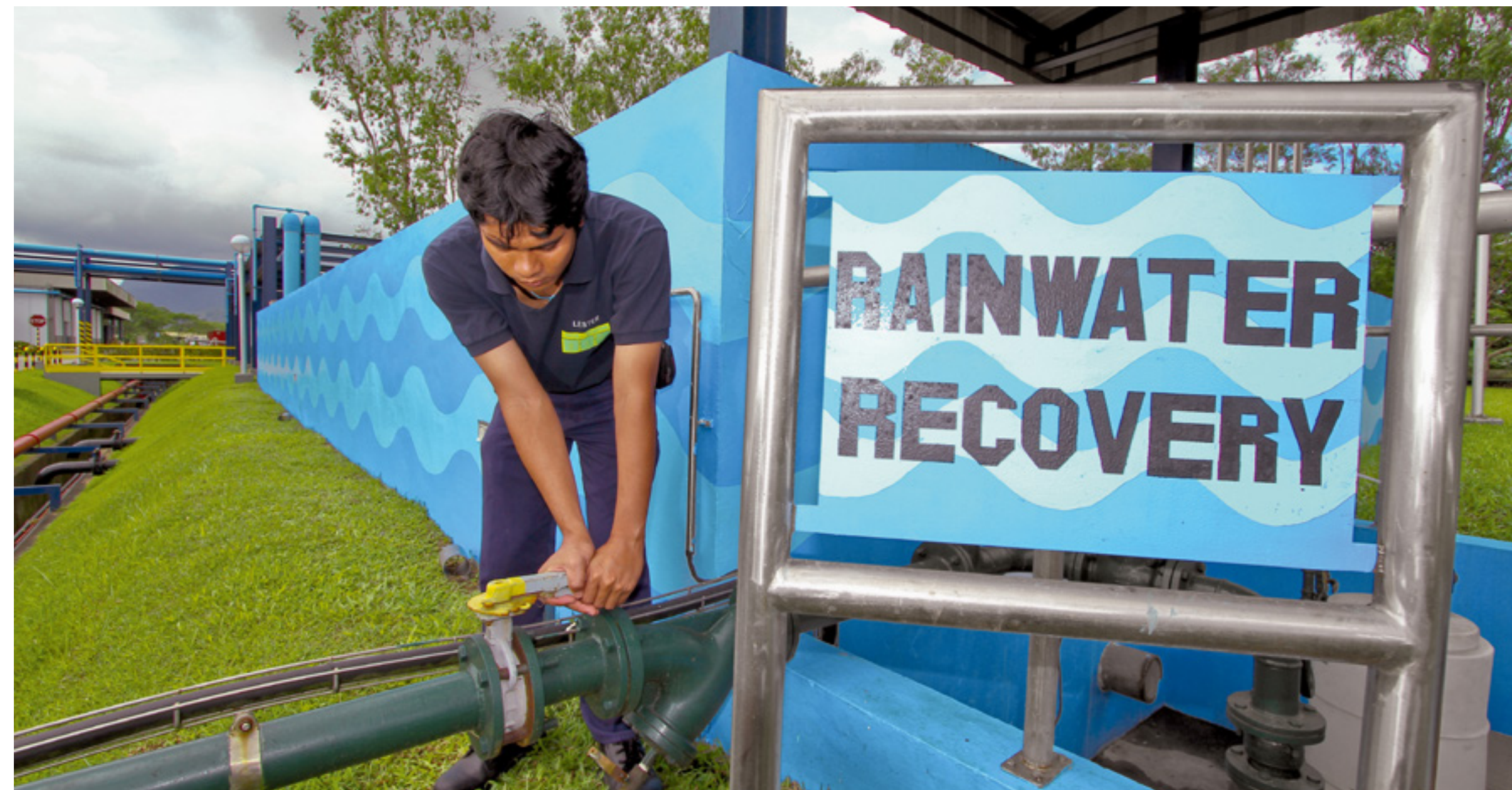
A rainwater collection system at our Lipa factory in the Philippines.
